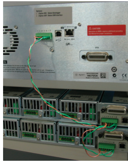
Figure 3b. Multiple mainframe wiring
