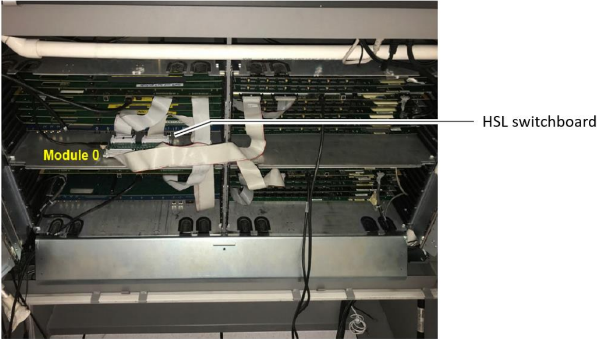
Figure 4. Location of HSL switchboard in an offline four-module i3070 system
